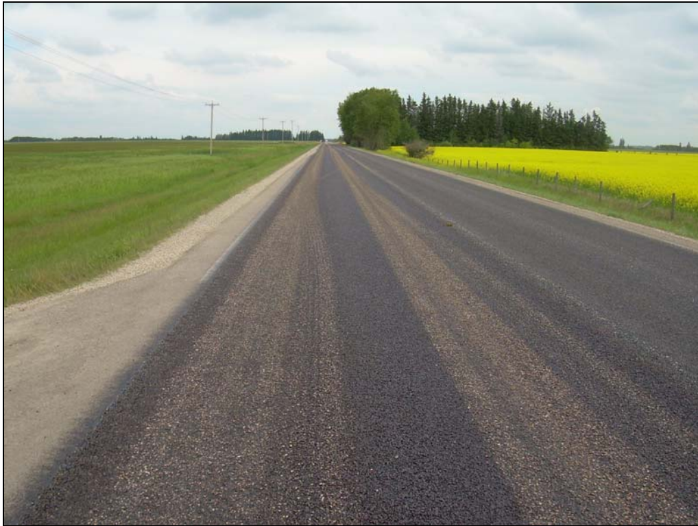
Photo 3. Tire Tracking on Insufficiently Cured Fog Seal
