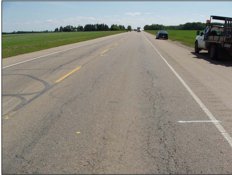
Photo 4. Hwy 39:10 - Extensive Wheel Path Cracking of Slight Severity
