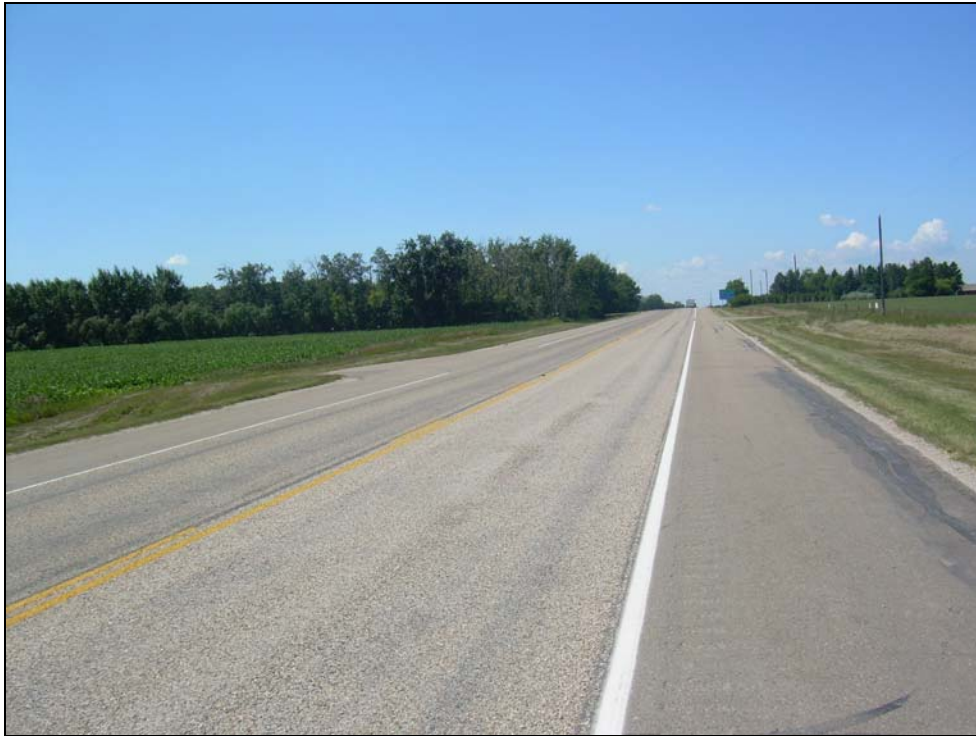
Photo 10. Racked-In Seal Coats – Without Fibres in Near Lane, With Fibres in Far Lane
